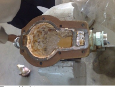
Figure No.24 Water trap valve body is covered with white solidified element (desiccant)
