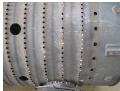
Figure No.7 Air passes blocked by white scale on combustion liner.
