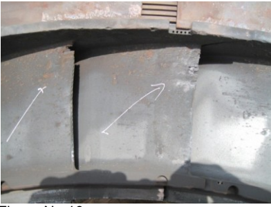
Figure No.16 First stage turbine nozzles bottom half, with signs of broken metal.
