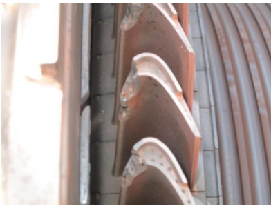
Figure No.18 Broken edges on first stage turbine bucket.
